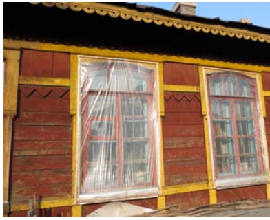
Fig. (1). Outer wall of a wood board house (photographed by authors themselves).
