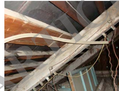
Fig. (12). Bending and sagging of wooden pole (photographed by authors themselves).
