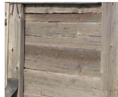
Fig. (8). Wood cracking (photographed by authors themselves).
