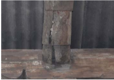
Fig. (9). Member cracking (photographed by authors themselves).
