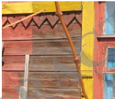
Fig. (7). Peeling of paint coating (photographed by authors themselves).
