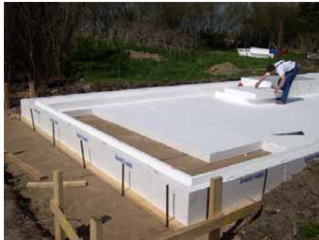
Fig. (5). a): prefabricated EPS elements mounted as the strip foundation and held together with large plastic securing clips, b): 0.3 m EPS, mounted as two layers on top of the base of stamped gravel bordered by the strip foundation, serving as the insulation layer beneath the concrete slab.
