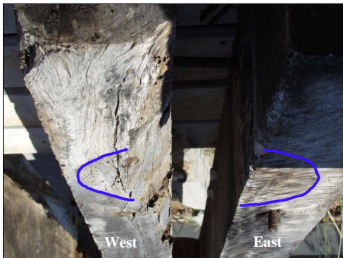
Fig. (14). Condition of the underside of the western half-cap on pier 1, pile 3.
