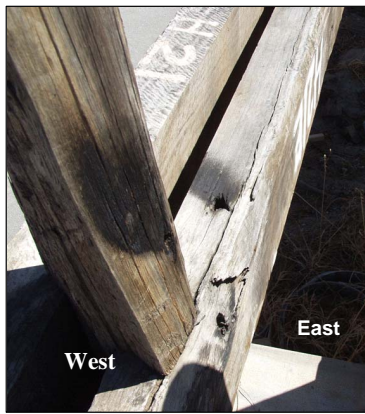
Fig. (16). Crack on the underside of the eastern half-cap at pier 21.
