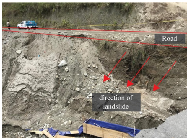
Fig. (1). The Bireuen-Takengon cross-road segment's experience of a landslide disaster, resulting in the collapse of a major section of the road.
