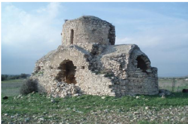
Fig. (4). Another example of the effect of a combination of forces acted on an abandoned byzantine monument in Cyprus, of which the seismic load is again the predominant force (Church of St. Marina near a village of the Larnaca district).
