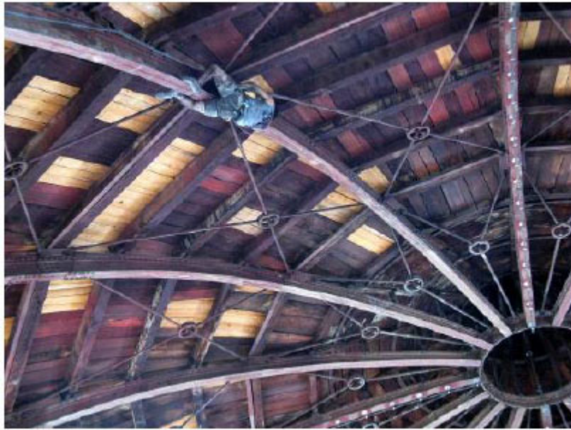
Fig. (13). Instrumentation of the dome with the help of a rock climber.
