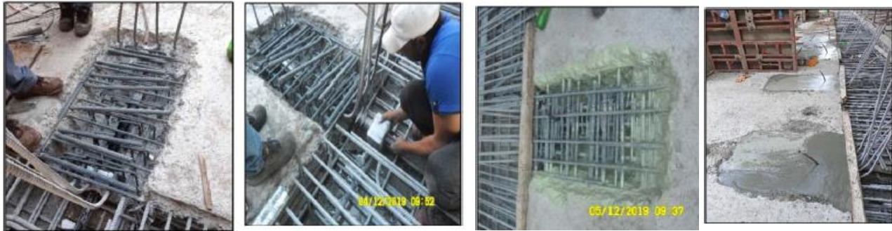
a) Breaking up concrete b) Replacing Post-tension System c) Cleaning and painting steel reinforcement with rich Zinc d) Casting with Rendorec LAXtra material
