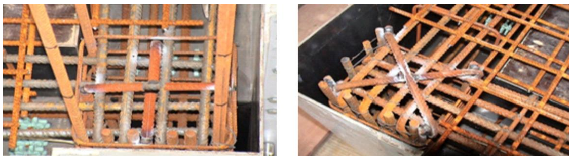
Fig. (2b). As built details of anchorage of column bars at the top of the storey joints, after Chaudat et al. [11].
