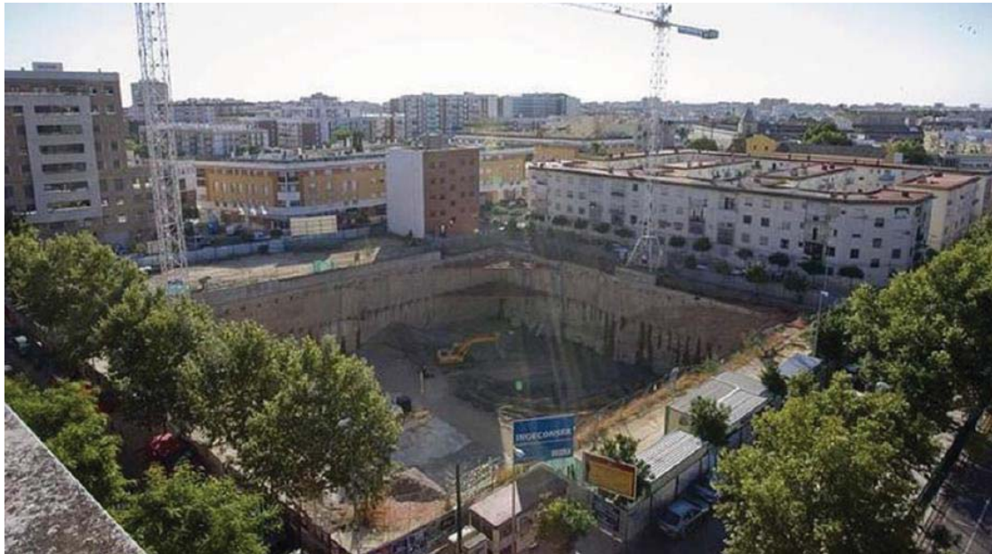
Fig. (2). Condition of the work on the day of the accident.
