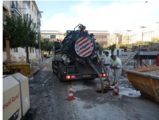
Pressurized-water cleaning truck
