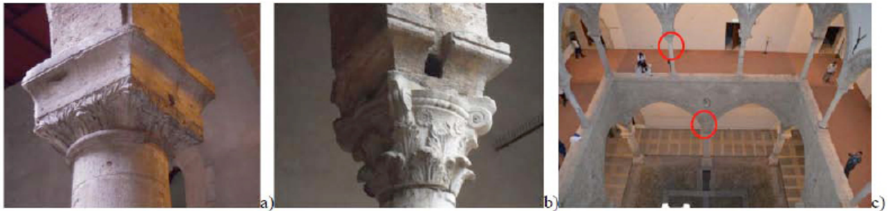
Fig. (9). Example of column capitals: (a) portico calcarenite capital; (b) loggia marble capital; (c) location within the courtyard.
