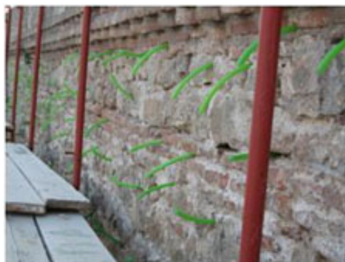
Fig. (17). Installation of a rubber tubes in the wall for the installment of the grout [3].
