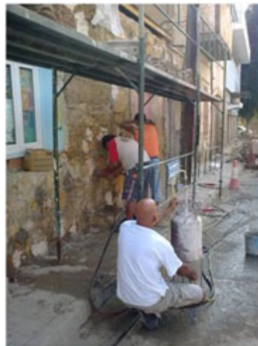
Fig. (19). An overflow of grout from holes at a higher level [3].
